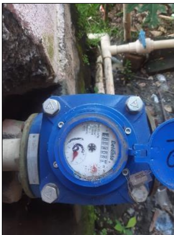
Figure 4-20: Sample photo of flow meter
