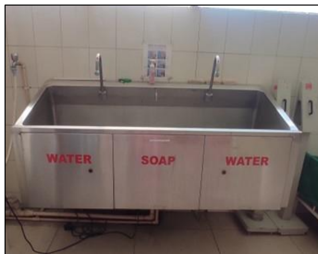
Figure 5-17: Sensors based wash basin
