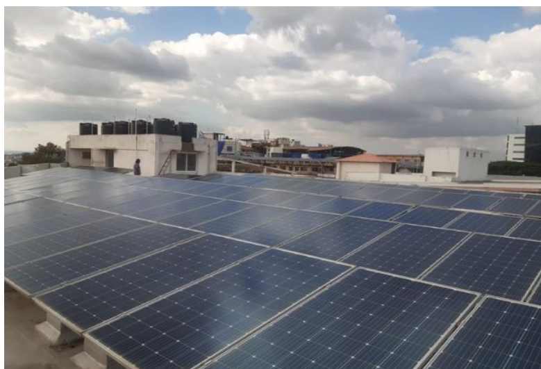
Figure 5-6: Solar rooftop PV system
