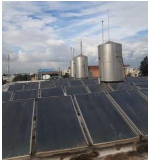
Figure 4-13: Hot water system in hostel
