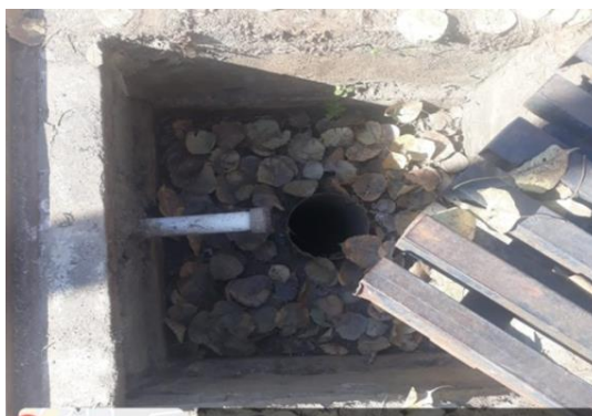
Figure 4-9: Rain water harvesting Percolation pit
