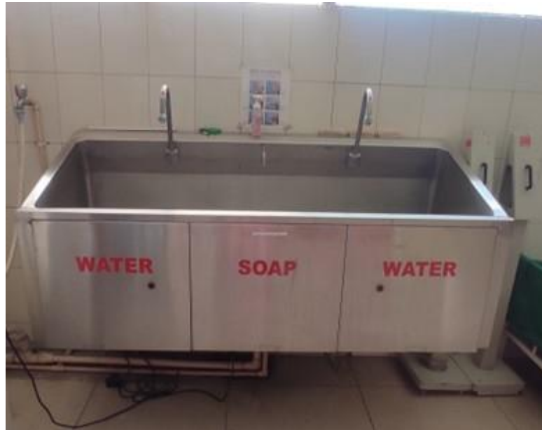
Figure 4-19: Sensors based wash basin
