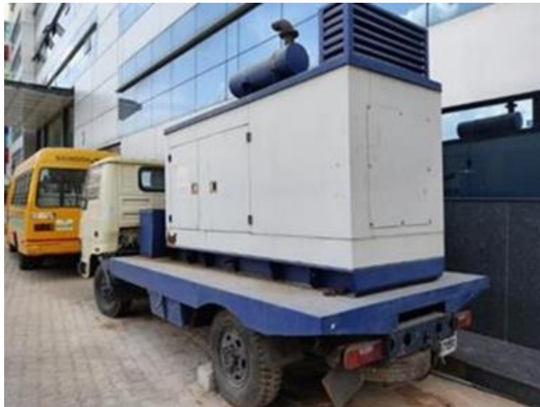
Figure 5-5: Mobile Diesel Generator (DG) set
