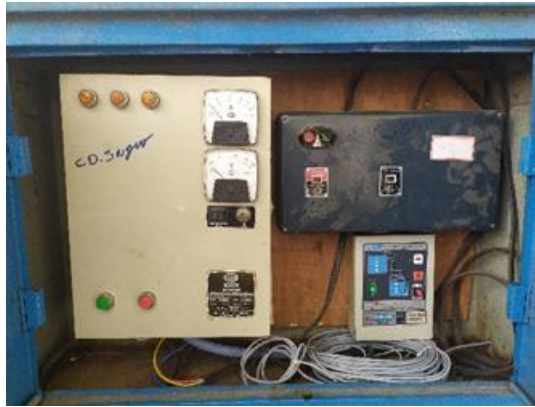
Figure 4-3: Level controller switch
