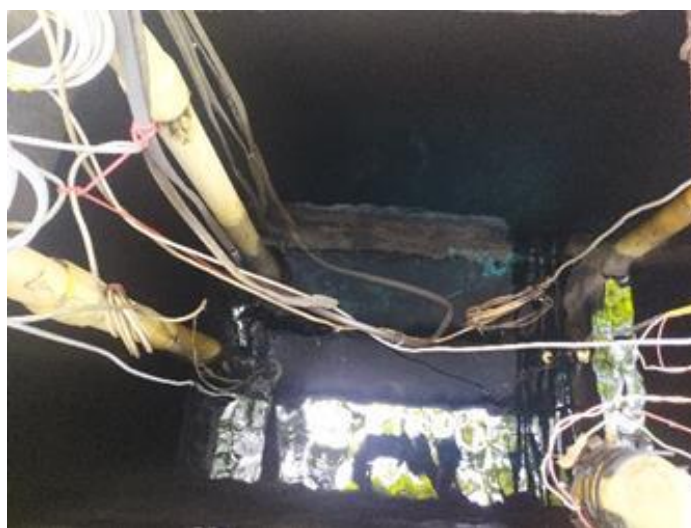
Figure 4-1: Raw water sump level controller
