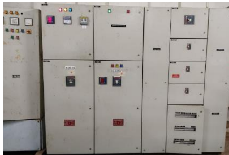
Figure 5-2: Electrical Panel Room
