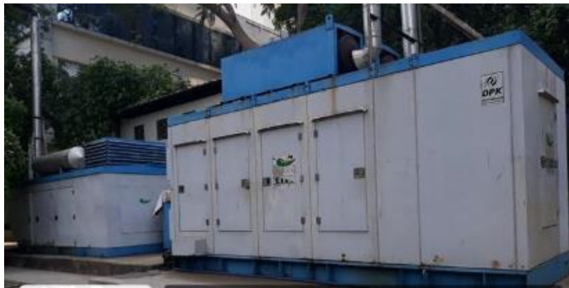
Figure 5-4: 400kVA and 250 kVA Diesel Generator (DG) set
