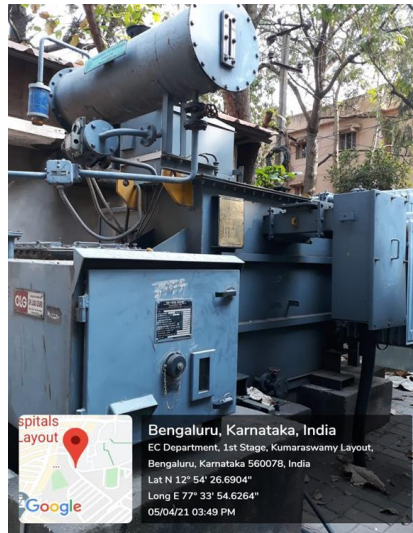
Figure 5-1: Transformer unit Installed in the campus
