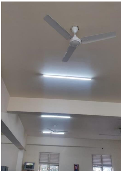
Figure 5-13: LED lights in Classrooms, Labs, and Corridors
