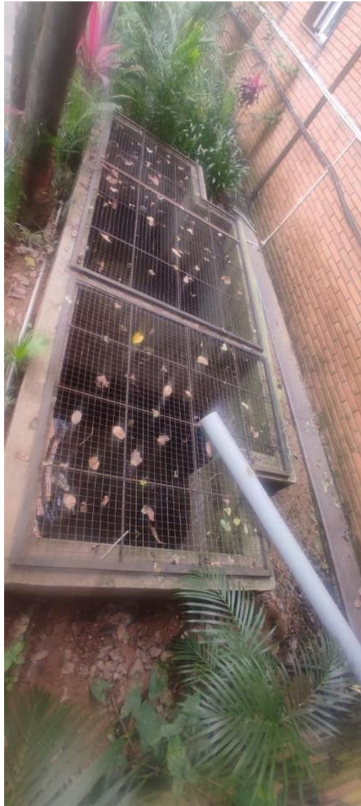
Figure 4-11: RWH sump near dental blocks
