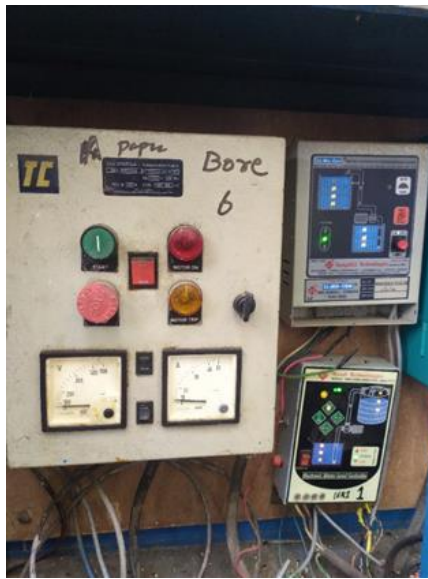
Figure 4-4: Bore-well pump panel and level controller switch
