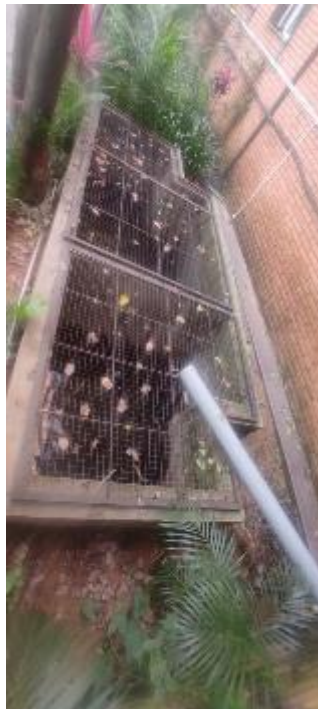
Figure 4-23: RWH sump near dental blocks
